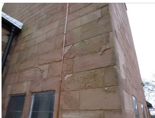
Delaminated sandstone to church tower
