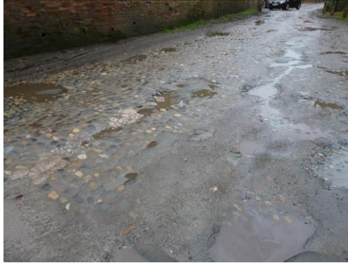
Uneven and partially covered stone sett surface
