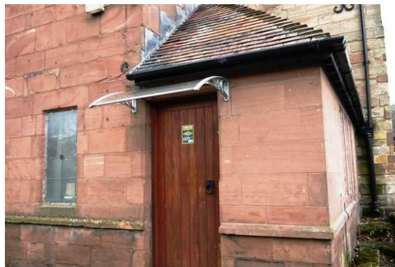
Inappropriate detailing on the church
